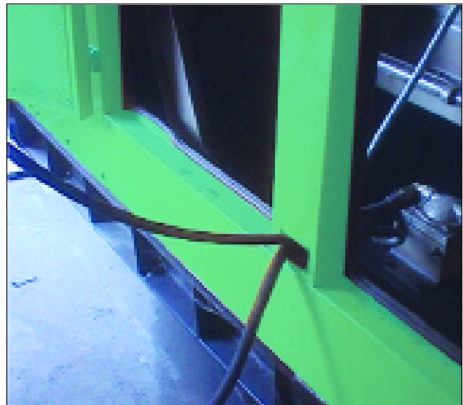
Poor routing of fuel hoses
